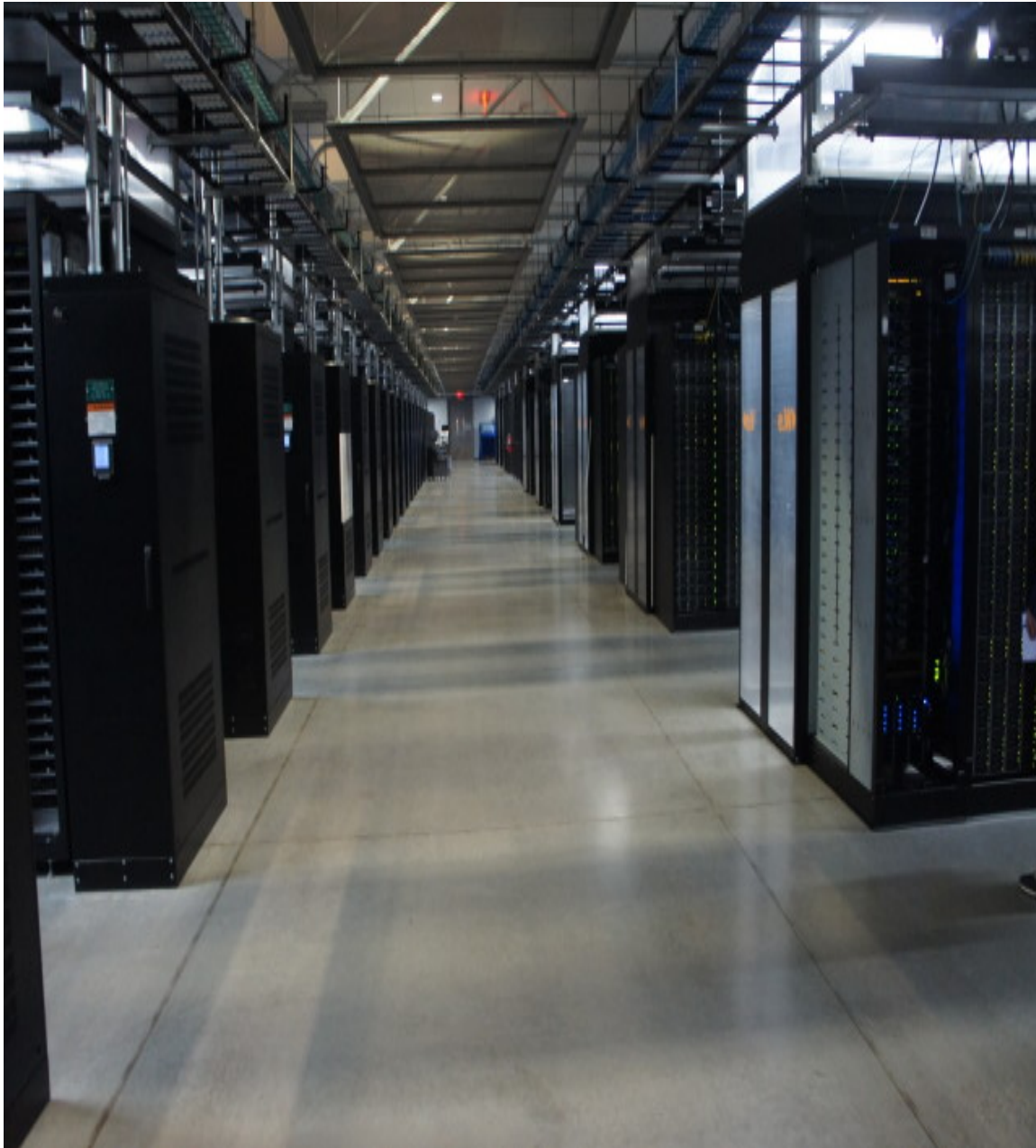
Figure 1. Server room (Fehrenbacher, 2012).
